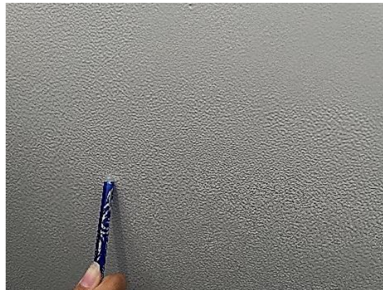
Gambar 6. Defect Orange Peel
